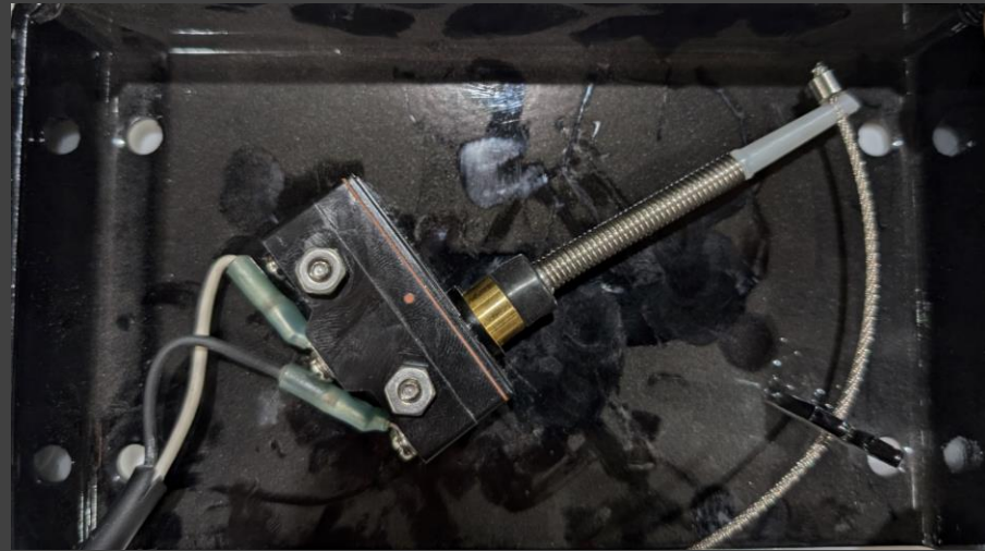
A2B condition: No tension on wire connected to wand switch and wand switch not actuated
